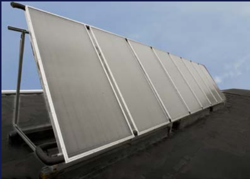
Circuits' rooftop solar panels heat 10 gallons water per minute to 70°F with as little as 3 ½ hours average daily sunlight
